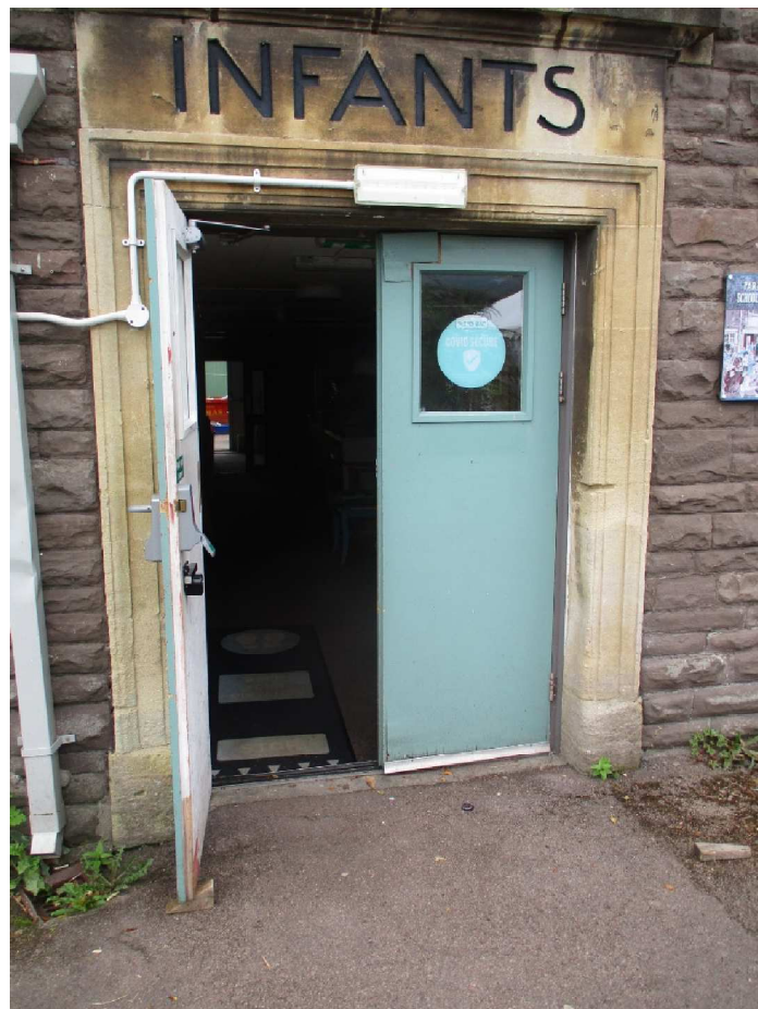
Photo 17 Raised threshold/ narrow entrance doors on route to Changing Places WC.
