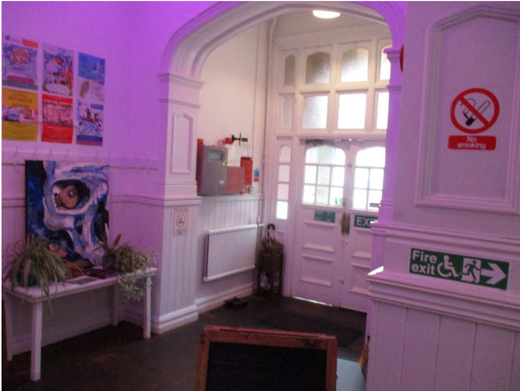
Photo 13 – Main entrance with stepped access. No refuge area to provide alternative egress route for wheelchair users.
