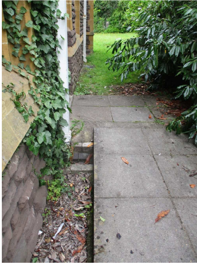
Photo 9 – Drop off at edge of path.
